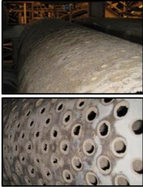
Figures 4 and 5: Struvite accumulation on a belt filter press drum before (top photo) and after (bottom photo) 5 months of HydroFLOW™ operation at the Orlando, Florida, Water Conserv II Water Reclamation Facility. Source: Miller et al., 2017.
