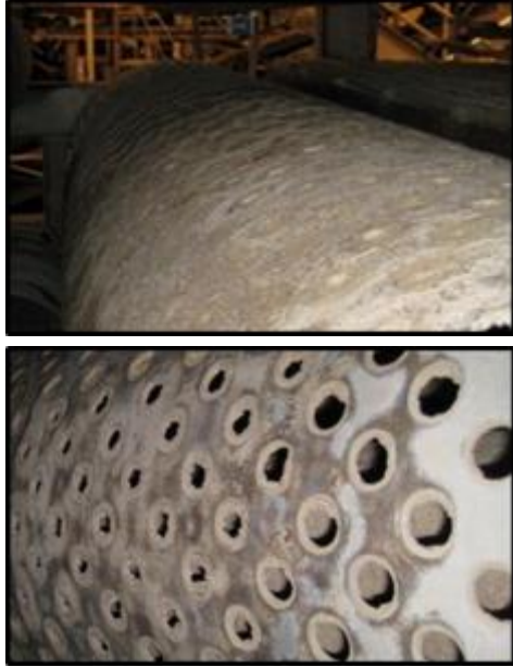
Figures 4 and 5: Struvite accumulation on a belt filter press drum before (top photo) and after (bottom photo) 5 months of HydroFLOW™ operation at the Orlando, Florida, Water Conserv II Water Reclamation Facility. Source: Miller et al., 2017.
