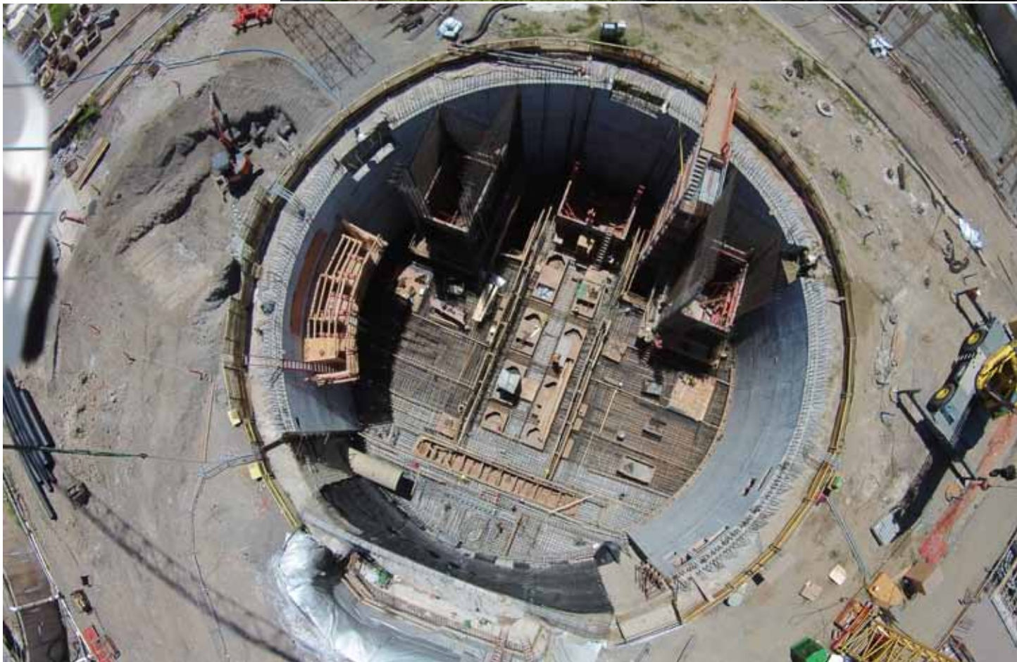
A new tunnel influent pump station shaft has been constructed as part of the Kaneohe-Kailua Wastewater Conveyance and Treatment Facilities Project. Bowers + Kubota
