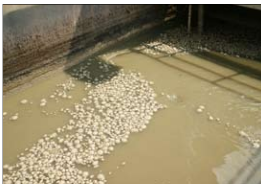
Grease balls like the ones pictured here form in the headworks of a wastewater treatment plant and periodically must be manually removed.
