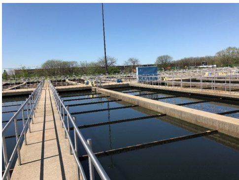
Figure 3— Rectangular Clarifier Configuration (PWD Southwest WPCP, PA)
