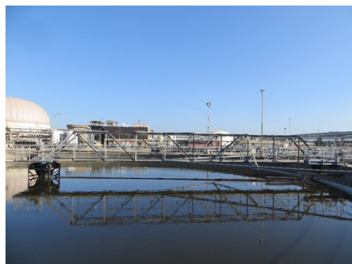
Figure 2— Circular Peripheral Feed Clarifier with Peripheral Overflow (East Bay MUD, CA)
