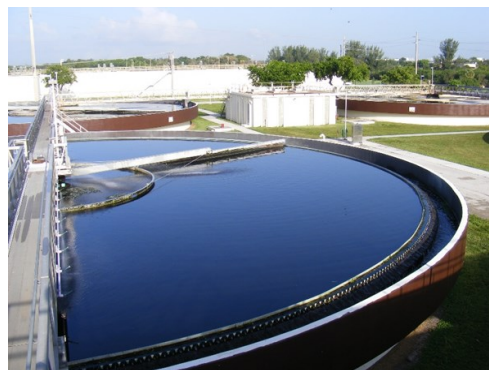
Figure 1— Circular Center Feed Clarifier with Peripheral Overflow (Broward County NRWTP, FL)
