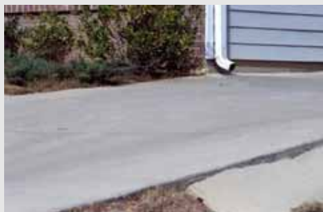
A directly connected roof drain
