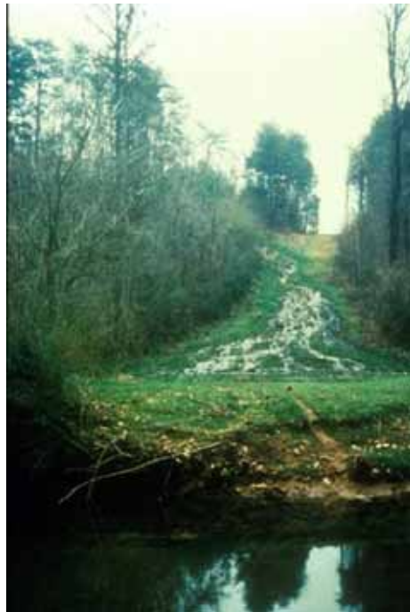
Sewage from clogged system overflowing into storm drainage system. SOURCE: Robert Pitt.
