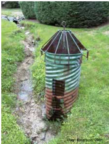
FIGURE 5-50 Rusted outlet structure. SOURCE: Reprinted, with permission, from Emerson. Copyright by Clay Emerson.
