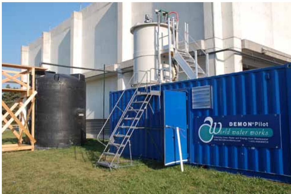
During the past few years, the Metropolitan Water Reclamation District of Greater Chicago has pilot tested a new sidestream nitrogen removal technology to help it prevent odor problems with transporting high-strength centrate from one facility to another. Chicago shared its findings through the Leaders Innovation Forum for Technology program. Water Environment Research Foundation
