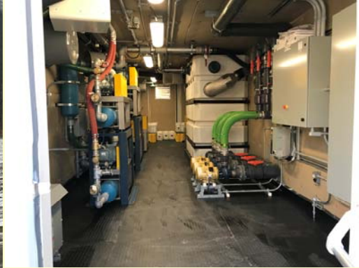
Blower and RAS Room
