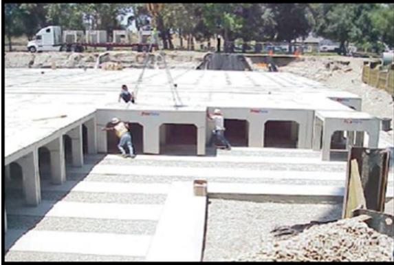
Photo 3: Installation of Sun Valley Infiltration Basins (Photo provided by LA County DPW)
