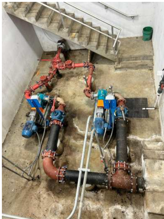
Figure E.6: DAF Tank 7-hp Pump
