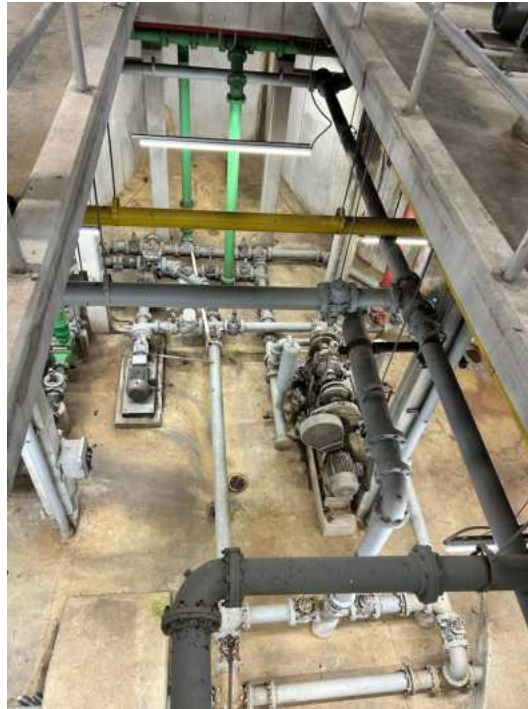
Figure E.7: Sludge Storage Tanks 15-hp Pump
