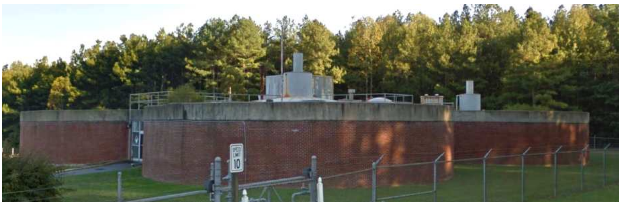
Figure 5.2.1: Current Anaerobic Digester Tanks Used as Sludge Holding Tanks
