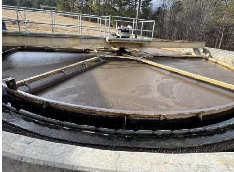
Figure 5.1.1: Current DAF Tank
